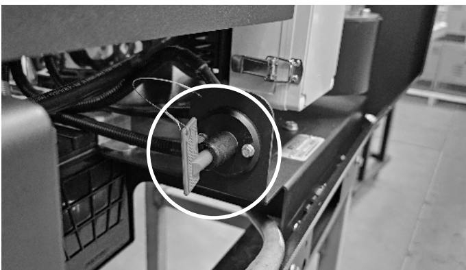
Figure.7 - Explorer G2 Battery Isolator
